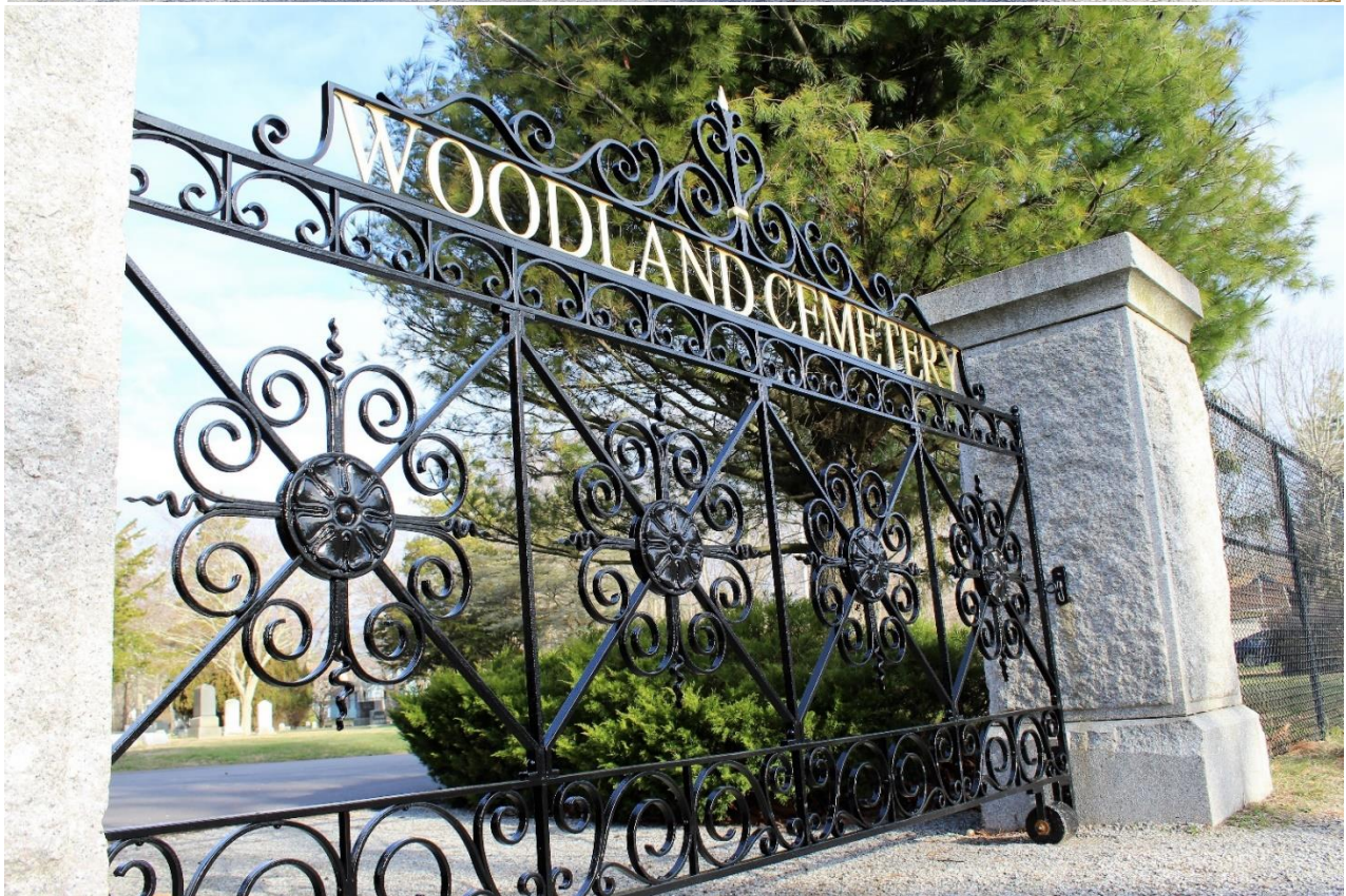
After many hours of extensive restoration by Spirit Ironworks, the Beautiful Woodland Cemetery Gate is ready again for decades of service.
