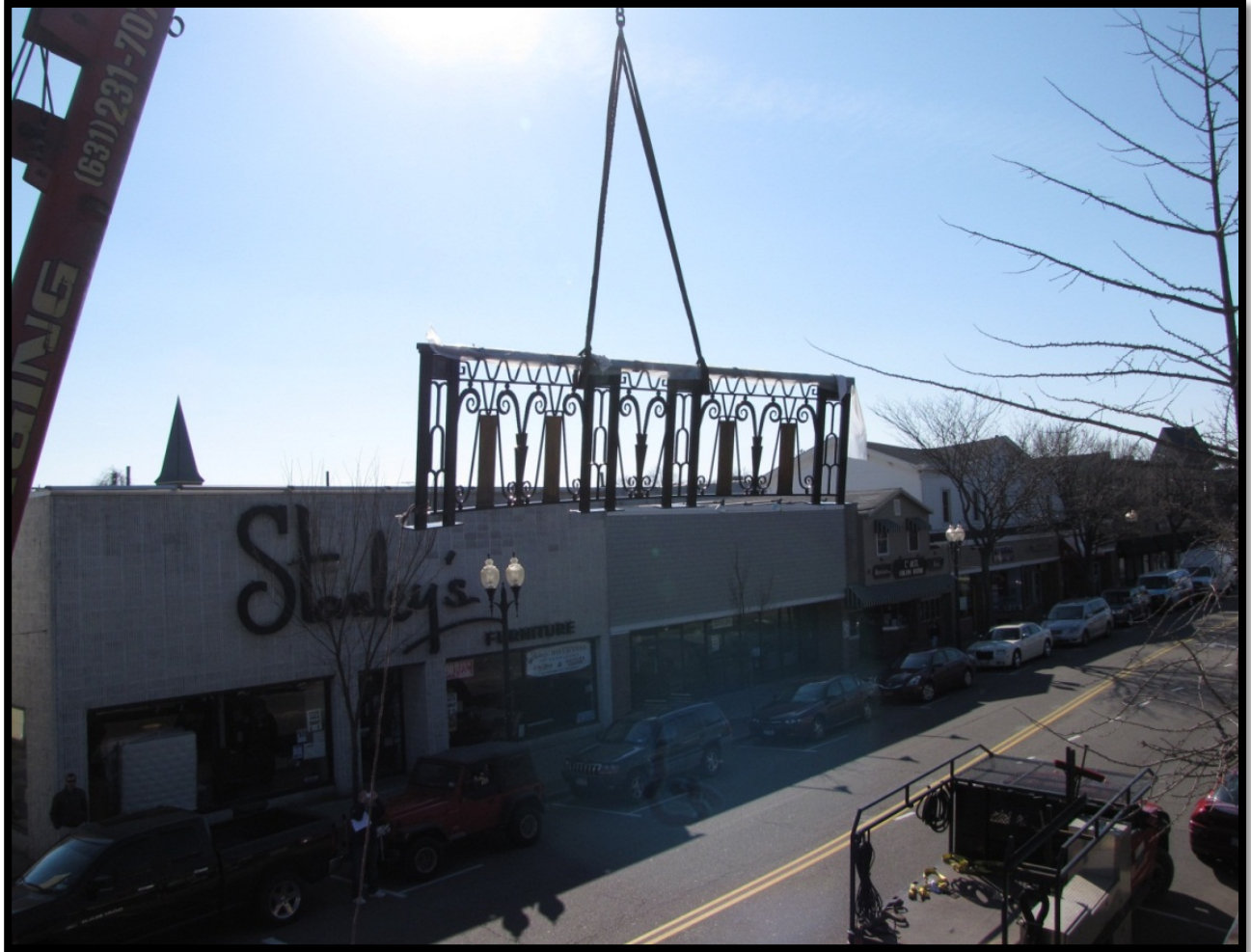
Here, the railing takes flight! Compliments of a local rigger. Our work truck and Main Street Patchogue in the background.
